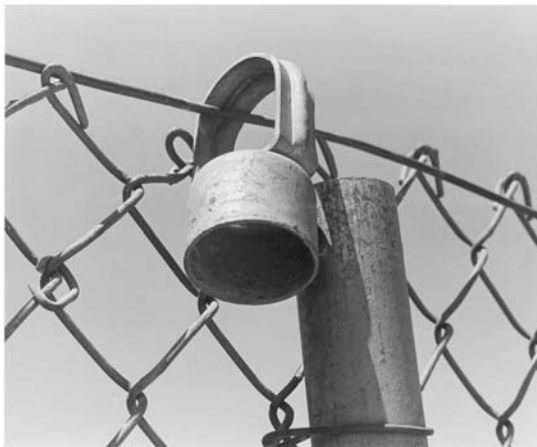
Figure 16 Mounting pole brackets for barbed wire, concertina or razor ribbon not properly secured to the fence posts
