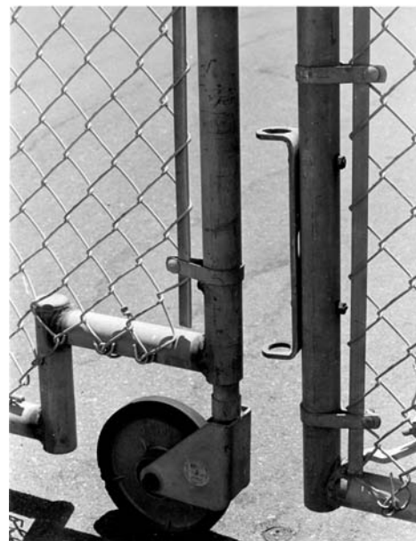
Figure 17 Missing vertical locking posts
