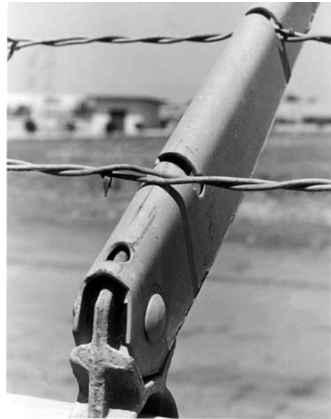
Figure 15 Barbed wire dangling due to missing keepers
