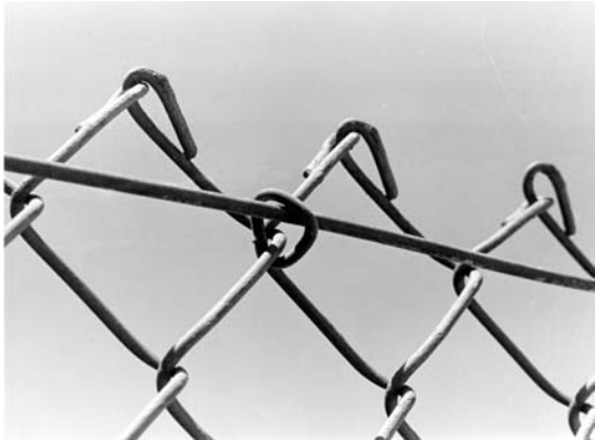
Figure 14 Loose fabric or clamp rings at steel wire stiffeners
