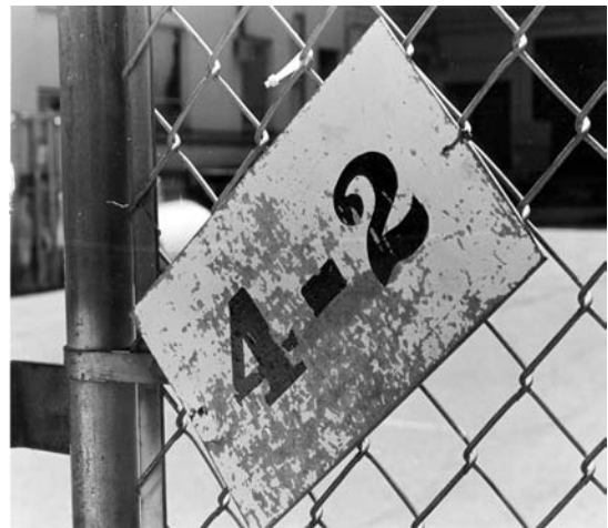
Figure 21 Signs and/or foreign objects not securely attached to the fence fabric or posts
