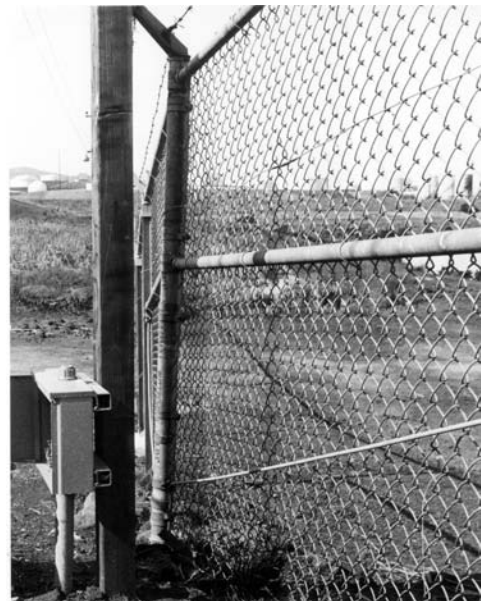
Figure 13 Loose fabric at diagonal stiffeners
