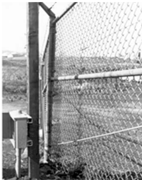
Figure 3 Loose fabric at diagonal stiffeners
