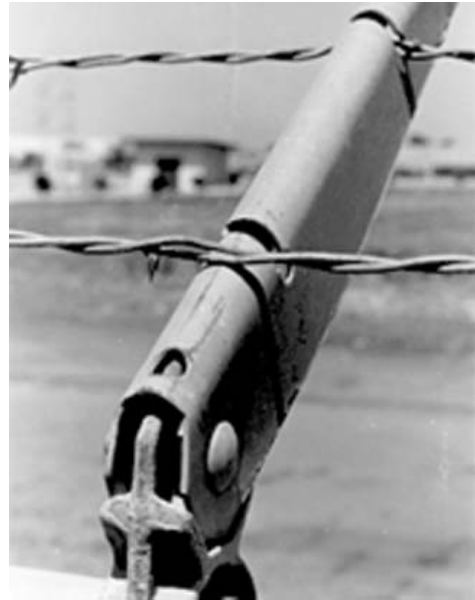
Figure 5 Barbed wire dangling due to missing keepers
