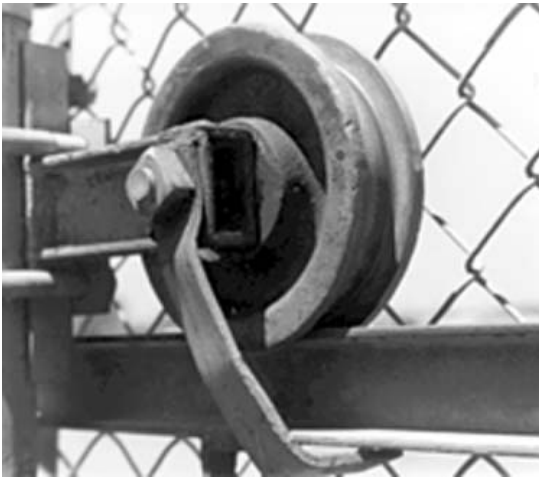
Figure 10 Too much play between rollers and rails
