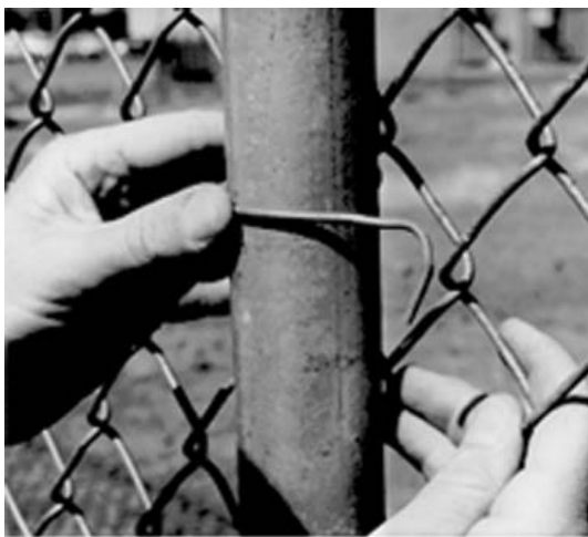
Figure 2 Loose fabric at fence posts or horizontal rails
