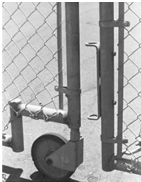
Figure 7 Missing vertical locking posts
