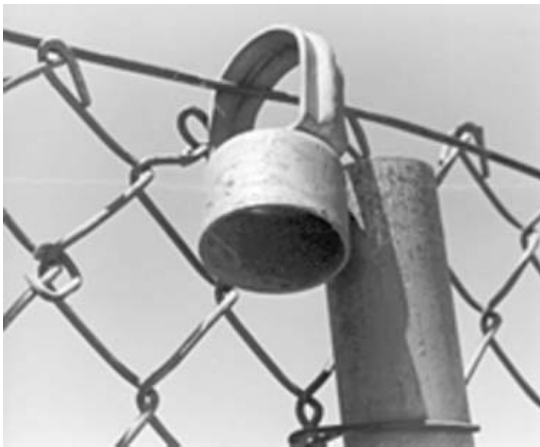
Figure 6 Mounting pole brackets for barbed wire, concertina or razor ribbon not properly secured to the fence posts
