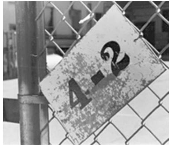
Figure 11 Signs and/or foreign objects not securely attached to the fence fabric or posts
