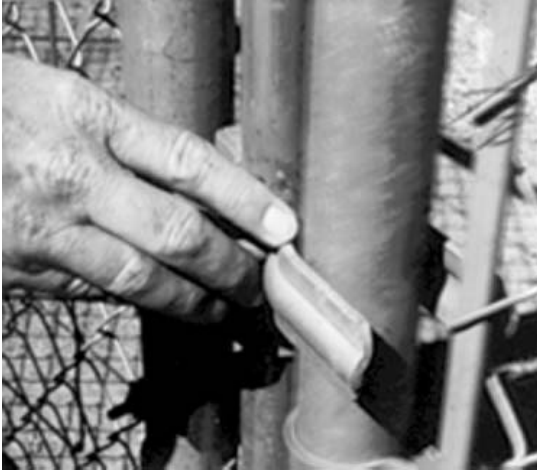
Figure 8 Excessive play between locking posts and metal insert
